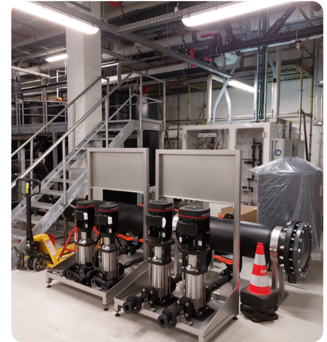
Water recovery plant (WRP)
